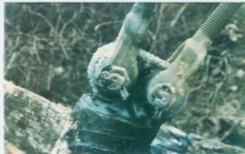
FX-763 Hydro-Ester Trowel Grade (water insensitive) is applied by hand with rubber gloves. Water is lubricant.
