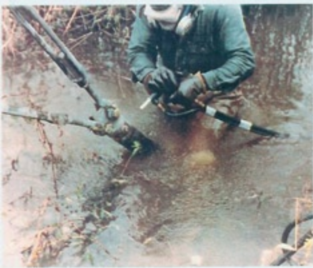
Sandblasting of anchor rod prior to installation of the FX-70® Inert Corrosion Free Sleeve System
