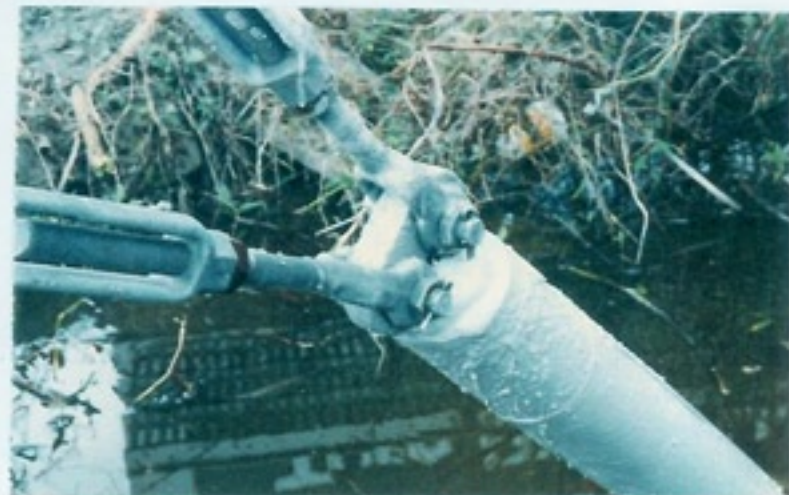
Completed encapsulation of anchor pad with FX-763 Hydro-Ester Trowel Grade and coated U. V. L. stabilization coating.
