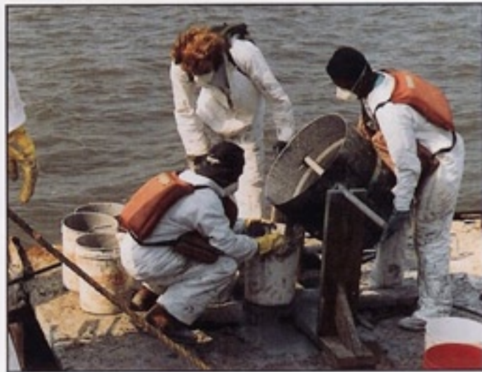
FX-70-6 Hydro-Ester® Pourable Epoxy Grout being mixed in drum, poured into pails to fill jacket.
