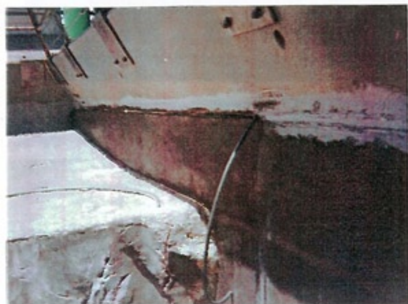
Inorganic cloth is tucked into kerf and sealed with FX-523 Flex-E-Pox to prevent edge raveling.
