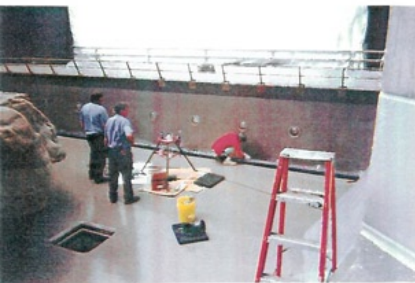
View of completed coating system. Anchors for surface mounted aerator system are secured into place using FX-763 Hydro Ester Trowel Grade Epoxy.
