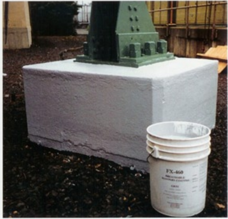
The remaining concrete bases are cleaned and protected with FX-460 Breathable Masonry Coating .
