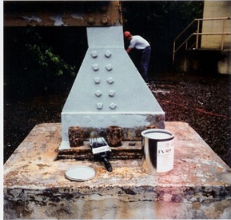
The steel tower supports are cleaned to remove peeling paint and primed with FX-509 Rust Inhibitive Primer .
