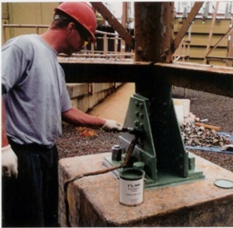
Two (2) coats of FX-509 Rust Inhibitive Coating are applied over the FX-509 Primer .
