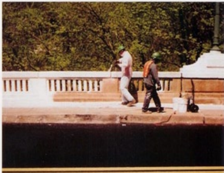
A Flanigan employee sprays FX-460 , as another checks on material. FX-460 can be rolled, brushed or sprayed at 200-300 square feet per gallon.
