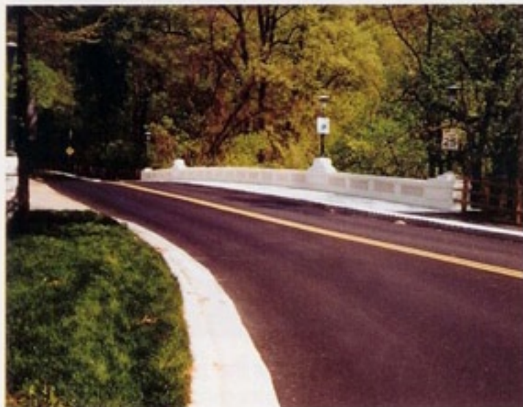
Windsor Mill Road Bridge over Gwynns Falls is revitalized using FX-460 Breathable Masonry Coating , Federal Color #27722, Beige
