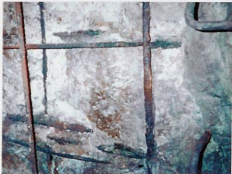
Severely deteriorated concrete ceilings and walls in steam vaults located beneath busy city streets.
