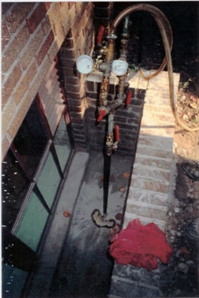
Gauges on the pump hoses allow the technicians to monitor the FX-III Jet Set during the pumping process.
