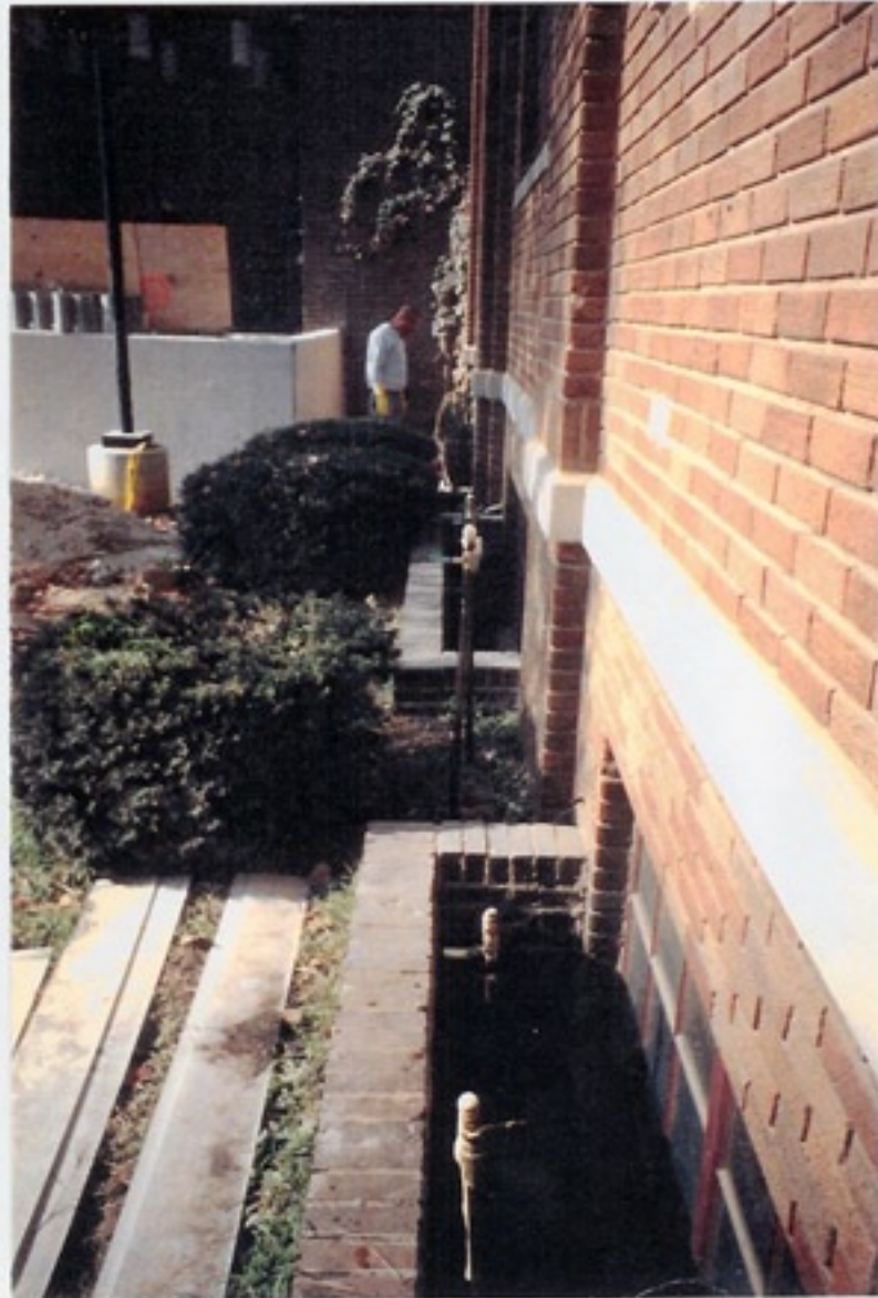
After all pipes have been pumped and removed, the pipe holes are patched with FX-922 Plug & Fast Set.
