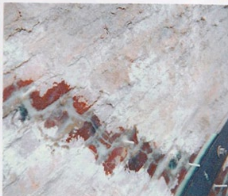
Injection ports are installed and secured in place with FX-763 Clear Non Sag Epoxy.
