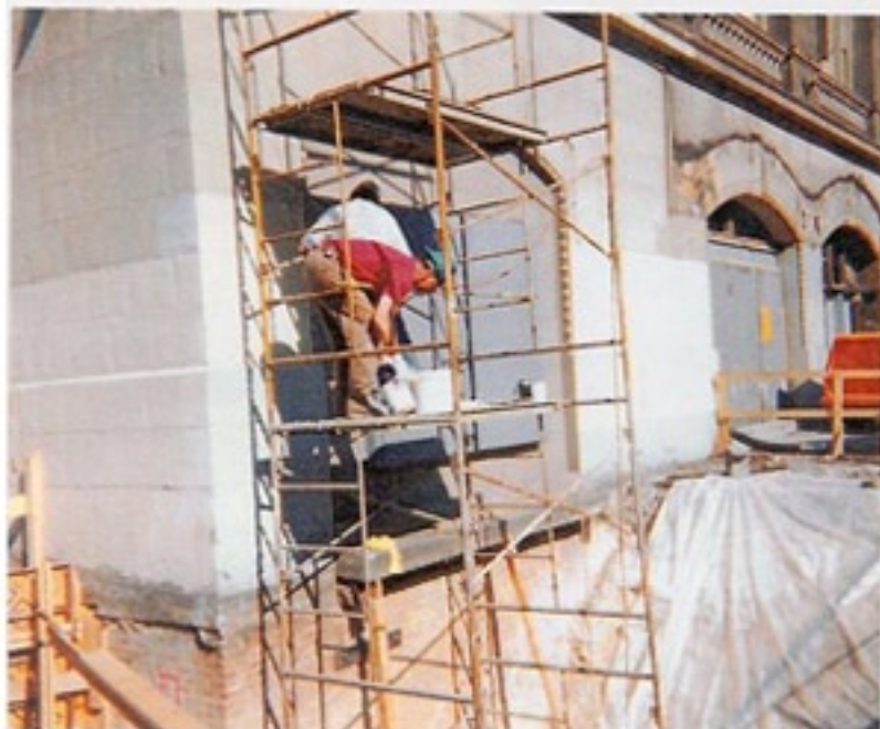
Cracks in the brick foundation wall of the Hippodrome Theater needed to be repaired.
