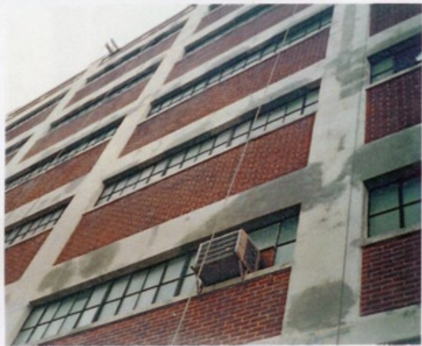
Repairs are complete and concrete is ready to have surface protection applied.
