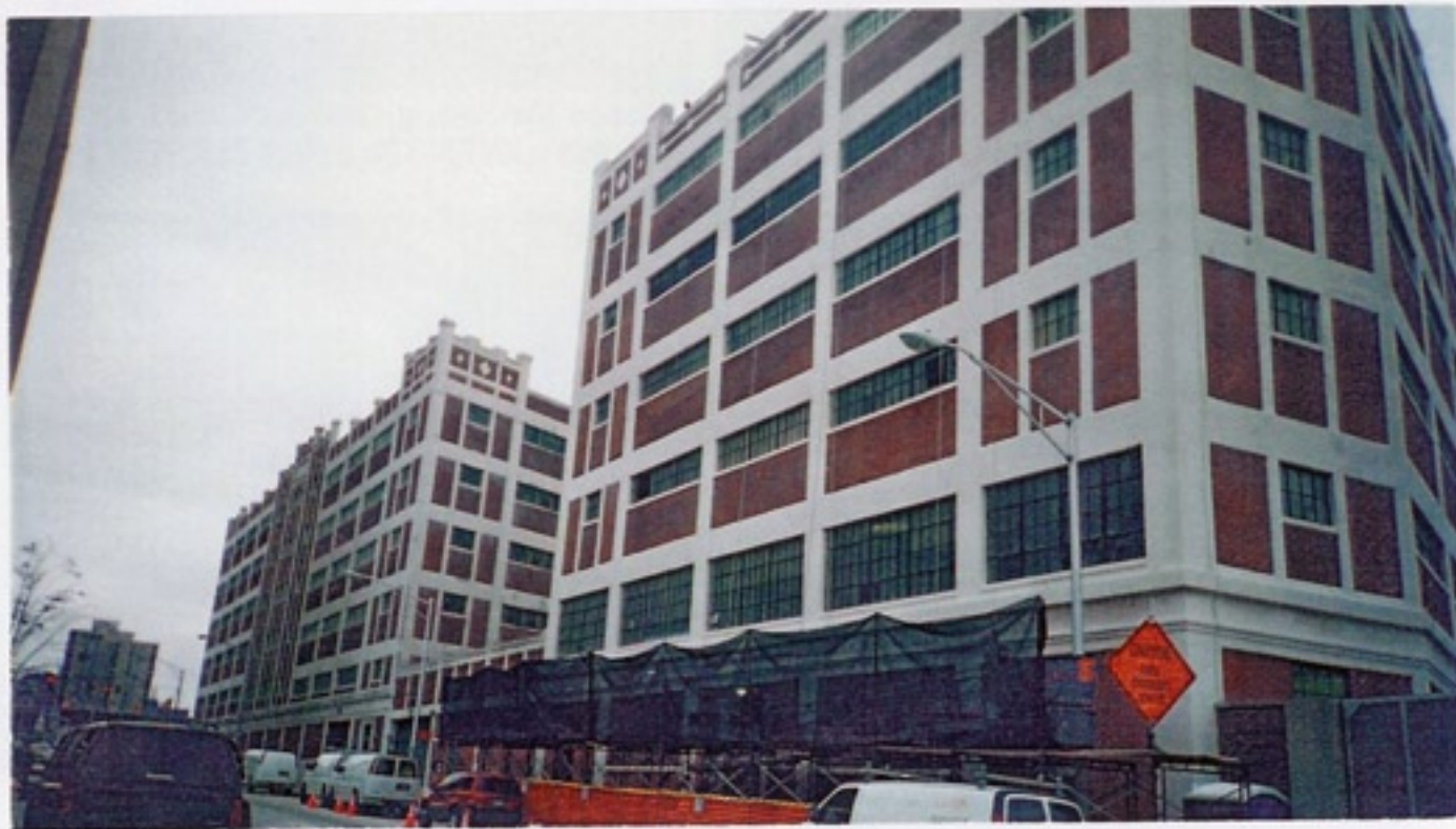
Concrete beams and columns are then protected and aesthetically enhanced using the FX-460 Breathable Masonry Coating System. The system provides long lasting high performance properties resulting from the unique, combination of water repellency and vapor permeability.
