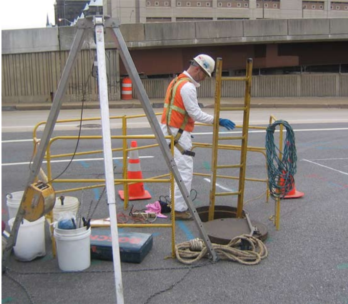
A broken sewer line leaking outside of a storm water manhole allowed raw sewage to infiltrate the walls of the manhole. FX-III Jet Set was needed to provide a waterproof barrier around the manhole to prevent additional contamination. Confined space safety equipment was required to enter the manhole.
