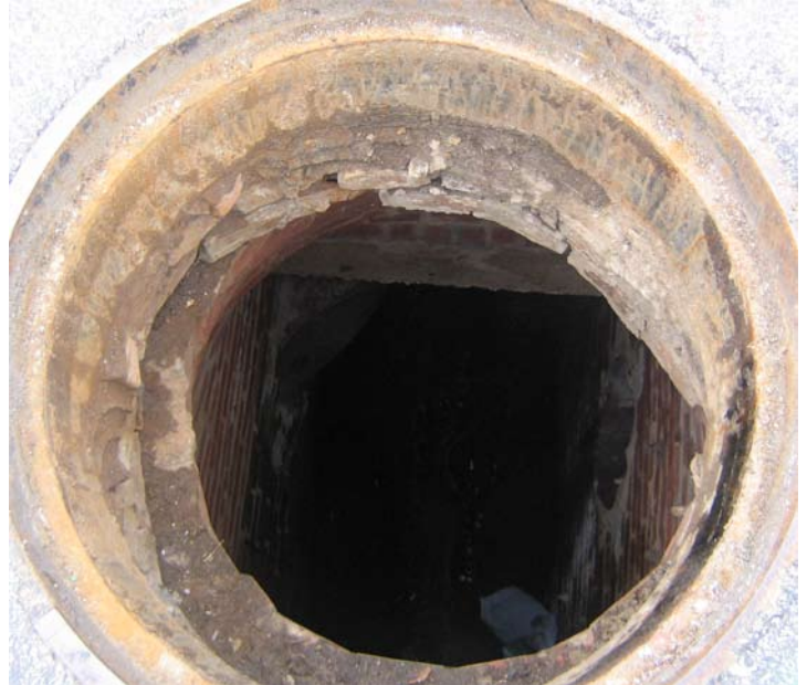
Deteriorated brick manholes are common throughout the USA. Aging infrastructure is a growing problem in the water-wastewater industry.
