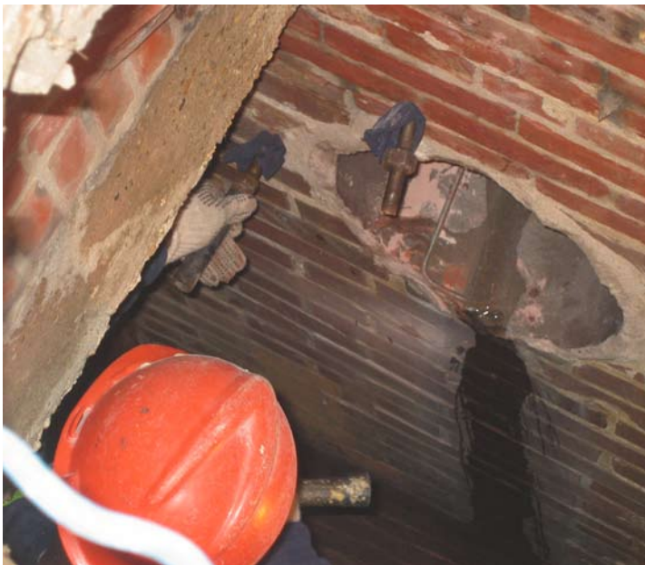
Prior to FX-III Jet Set application, holes were drilled through the brick walls to the outside of the manhole. Injection packers were placed into drilled holes.
