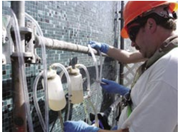
A worker monitors the injection process. The vacuum port is above, out of view from the camera
