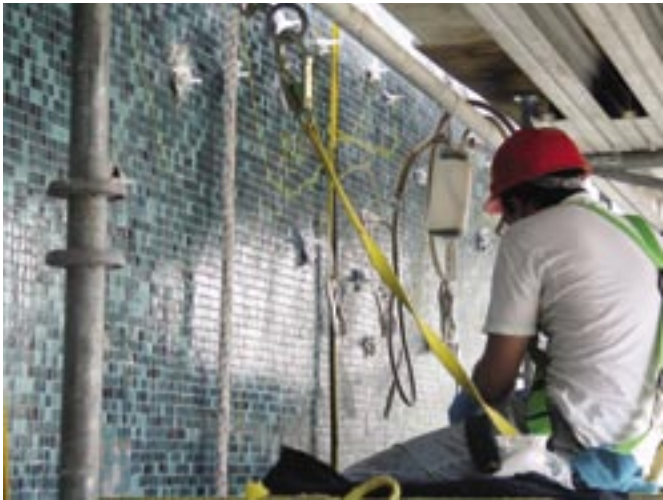
The layout of the MMA vacuum injection process. Note the clear tube inserted into the red port at the top of the photo. This hose is attached to the vacuum pump creating the vacuum at the top of the delamination. The bottle hanging from the railing contains a portland cement enhanced mixture of MMA that is being drawn into the wall at the white port. The process required hundreds of ports
