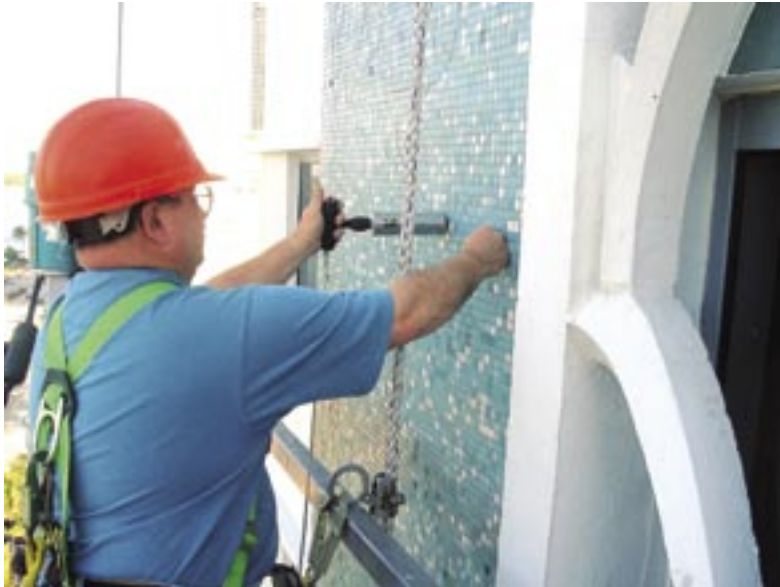
The impact echo testing in operation. The device demonstrated is the hammer sounding and transducer. Note the portion of the wall above the area being examined. The Xs on the wall indicate areas of delamination
