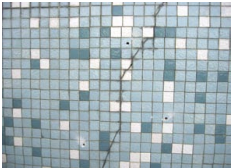
Layout of additional pins inserted for crack stitching
