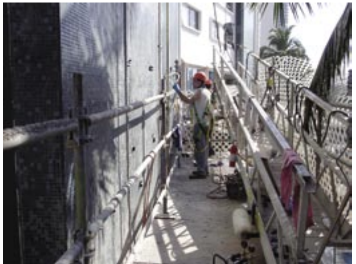
The vacuum process being performed at ground level. The vacuum pump is seen in the right center of the photo under the swing stage. A spare pump is seen at the bottom of the photo
